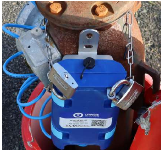
Installation with padlocks
