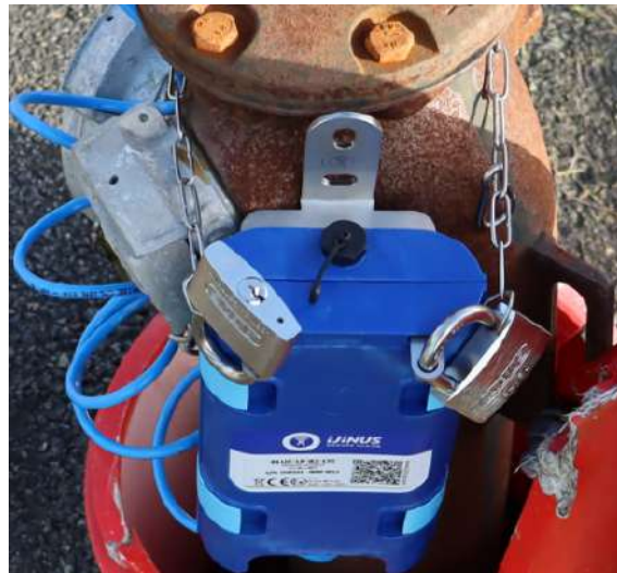
Installation with padlocks
