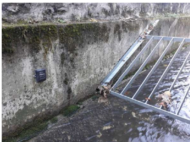
Installation for monitoring grid fouling
